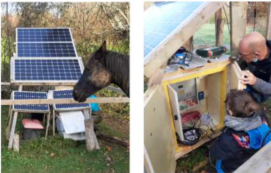
Fig. 3.15 DTS instrument and the solar panels powering its battery.
